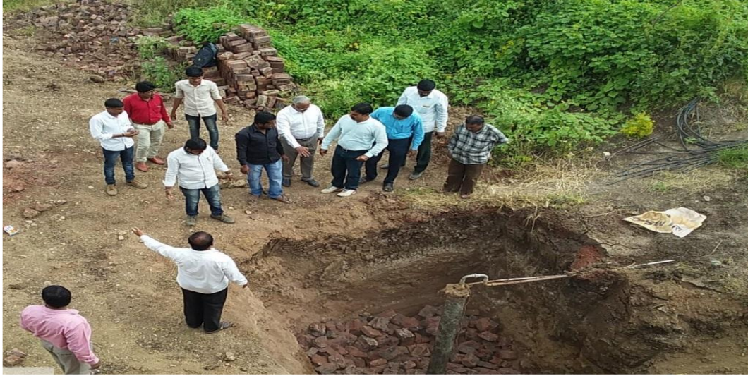
Roof Water Harvesting and Bore-well Recharge Project at Prof. Sambhajirao Kadam College, Deur (Date: 18.01.2020)
