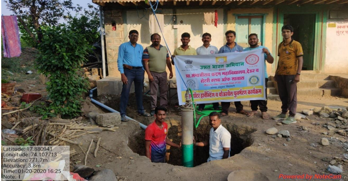
Rain water harvesting and Bore well Recharge, Place: Dahigaon (Tal. Koregaon, Dist. Satara)
