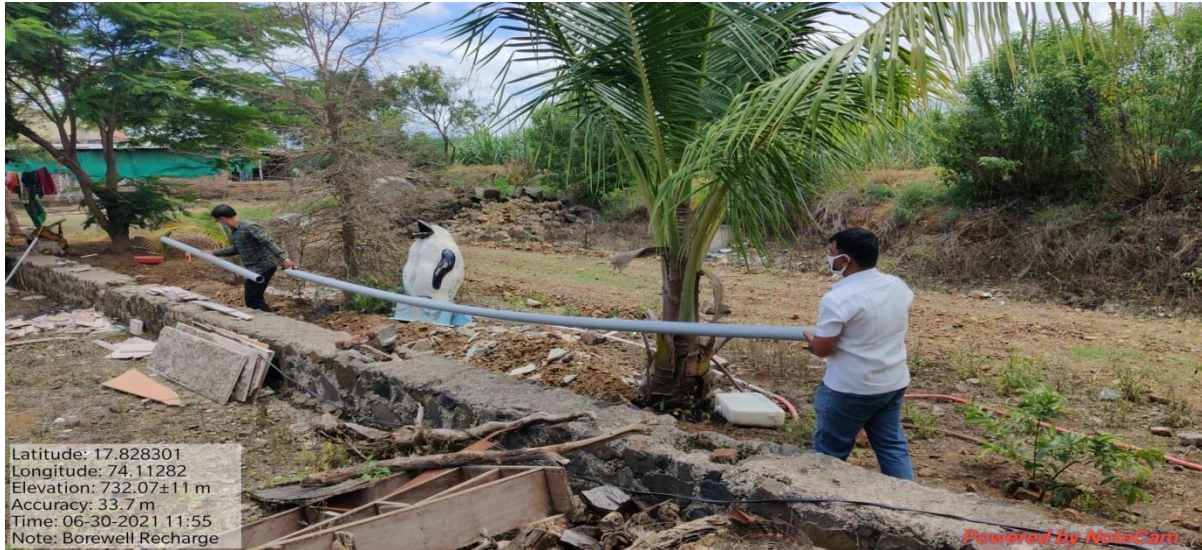
Roof Water Harvesting and Borewell Recharge Project (Datta Mandir, Palashi)
