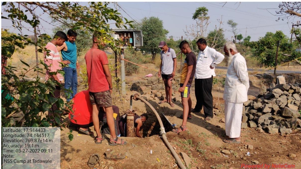
Rain water harvesting and Bore well Recharge, Place: Tadawale S.W., (Tal. Koregaon, Dist. Satara)
