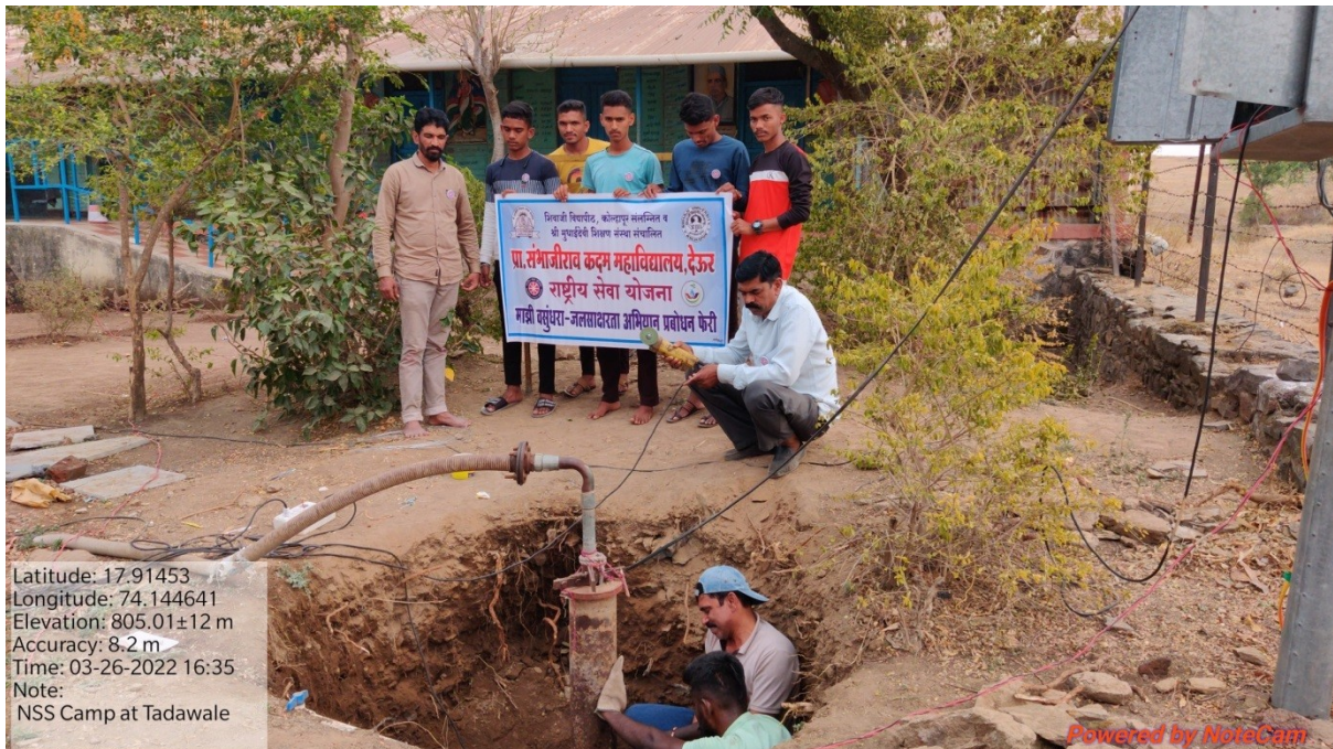
Rain water harvesting and Bore well Recharge, Place: Tadawale S.W., (Tal. Koregaon, Dist. Satara)
